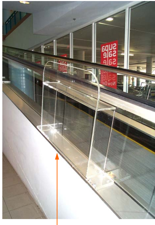
Large Guard on moving walkway
