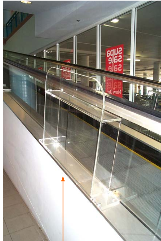
Large Guard on moving walkway
